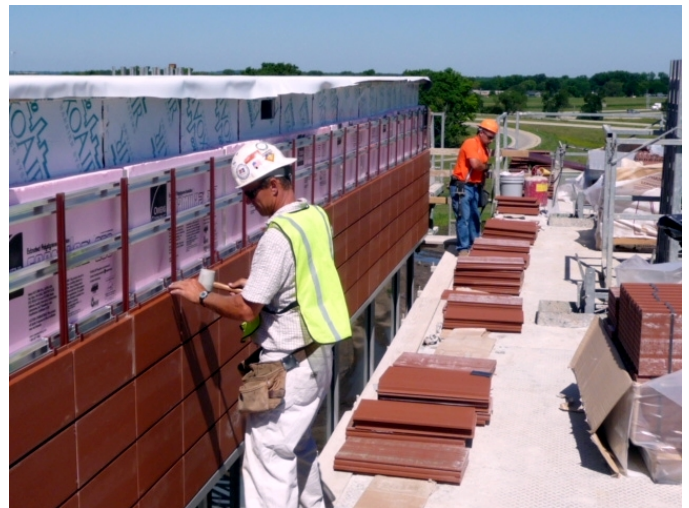
BAC mason contractors install the aluminum support system and the terra cotta facing units at the Kerry America headquarters in Madison, Wisconsin.
