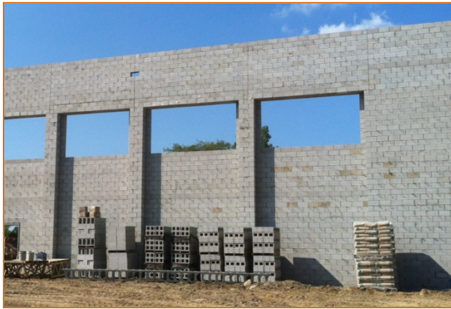
Photograph 2: Masonry walls under construction utilizing Internal Bracing. (Credit: Koch Masonry, Dexter, MI)
