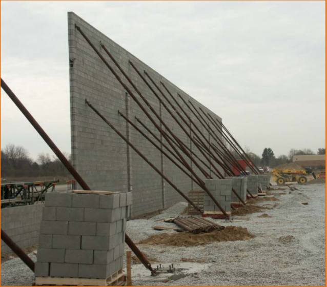
Photograph 1: External pipe braces utilized on a masonry wall under construction with anchorage to block pallet 'skids' and column foundations. (Credit: Davenport Masonry, Holt, MI)
