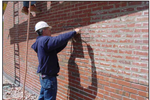
Apply the new prehydrated mortar in 1/4" lifts to minimize voids and air spaces that could lead to shrinkage of the mortar.
