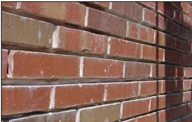
All deteriorated mortar must be removed so resultant joints have a uniform depth of 1/2" to 3/8", or until sound mortar is reached.
