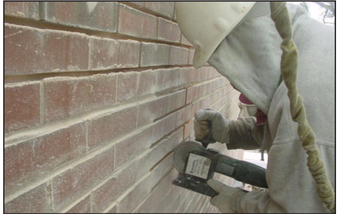
Union tuckpointers are trained to use care when using mechanical tools such as this grinder to remove deteriorated mortar, as not to damage the adjacent masonry units.
